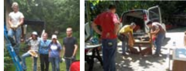
Two teams of youth and advisors traveled to KY to repair homes for the Appalachia Service Project
